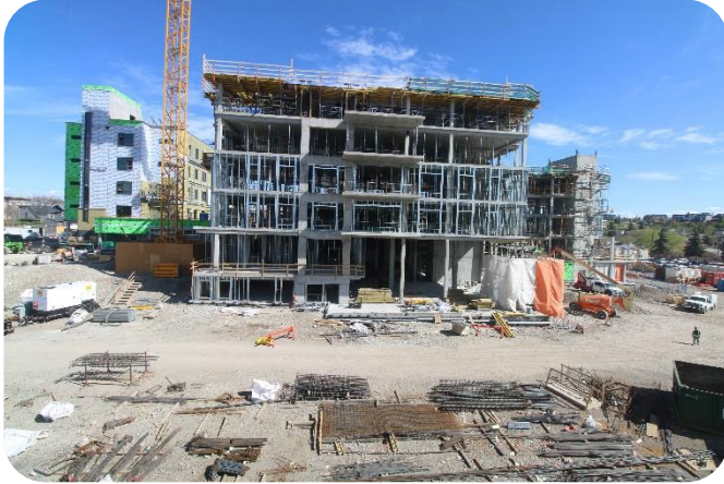
West tower concrete structure is complete and exterior framing in progress. Photo looking at South elevation of building.
