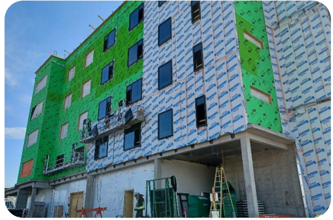
West tower envelope, windows, exterior framing and boarding is underway. Photo looking at West elevation of building.
