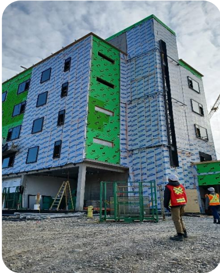
Southwest corner of building. Windows and vapour barrier being installed on exterior boarding.
