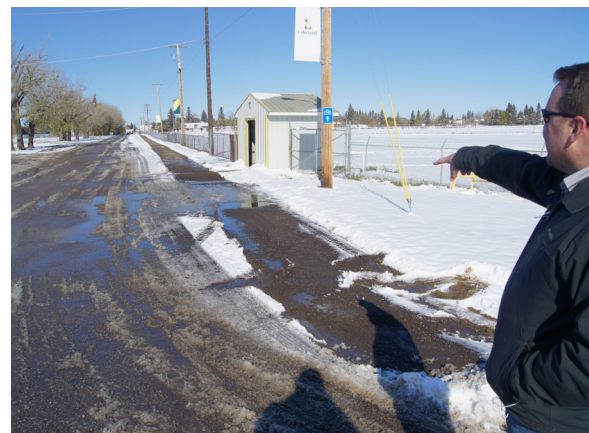
Figure 19: Demonstration of where pedestrian walkway is provided simply by clearing a path. Additional supports could be provided in paint and other designation to identify the space for walkers
