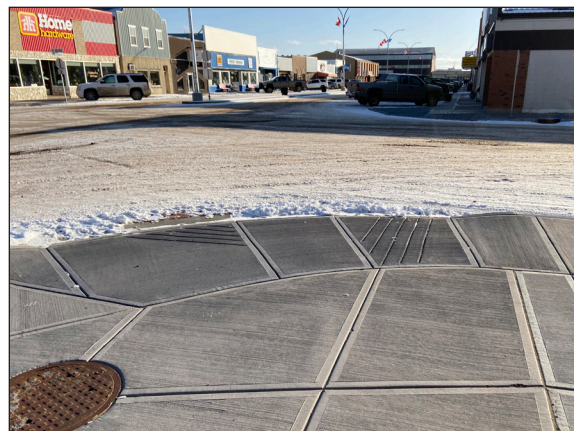
Figure 5: Example of crossing with a wide curb ramp that allows pedestrian to cross the street in all directions.
